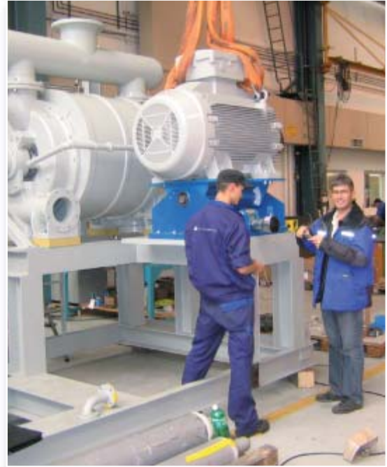
Installation of a 1750 kg heavy 250 kW motor on the Motorbase MB 100 and tensioning process of the eight SPC V-belts by the integrated bevel-gear shaft drive
